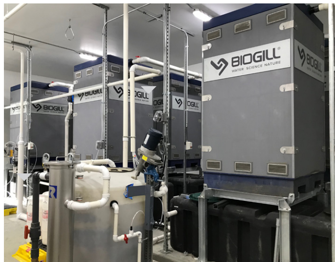
Six BioGill Tower units are used in the biological stage of the treatment process.
