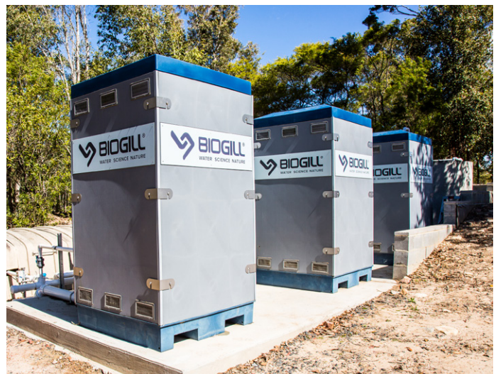
The BioGill system treating wastewater onsite.
