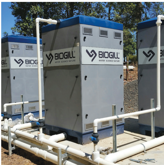
Retrofitting BioGill units saved the client money, increased the treatment performance and extended the life of the existing plant.
