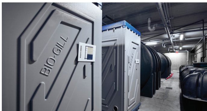
Four BioGill units operate at the winery.
